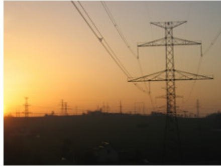
Fig 1. EHV overhead lines
