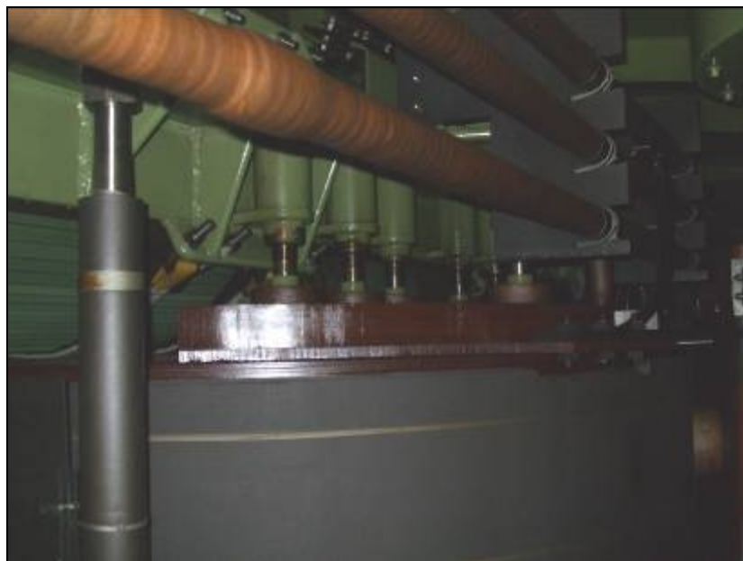
Figure 7 Photo from 2007 inspection, B/yellow phase HV side clamping bolts
