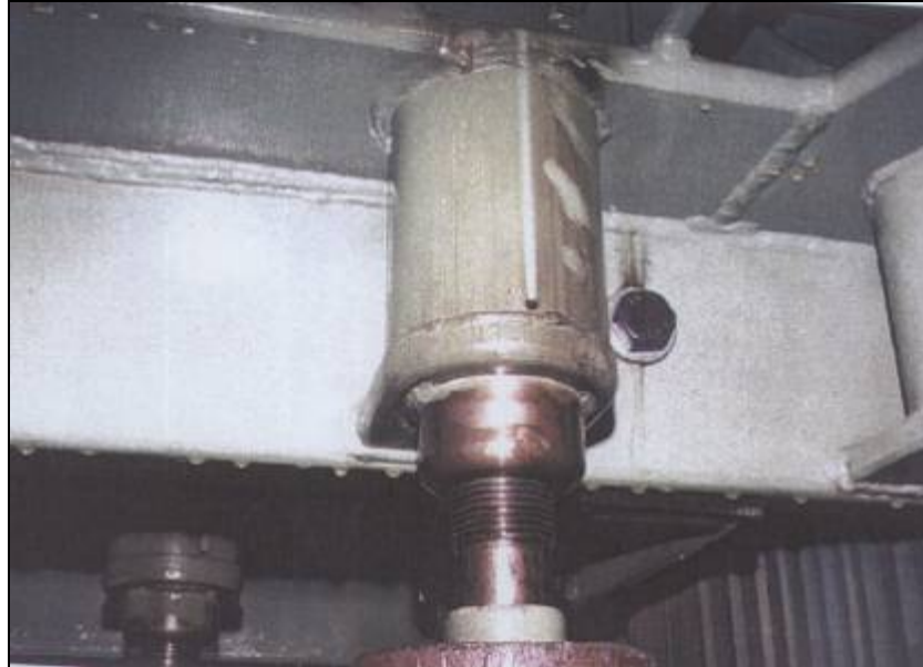
Figure 6 Photo from 2001 inspection of the transformer with carbon marks
