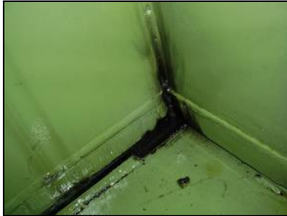
Figure 12 HV red phase inside corner
