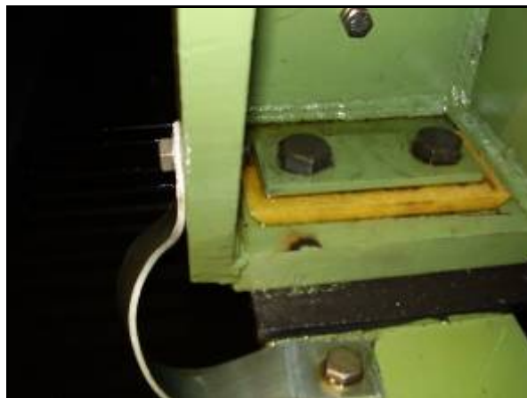
Figure 13 HV yellow phase left hand side
